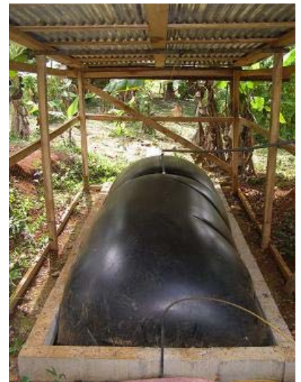
Hand constructed Biofuel Tank
